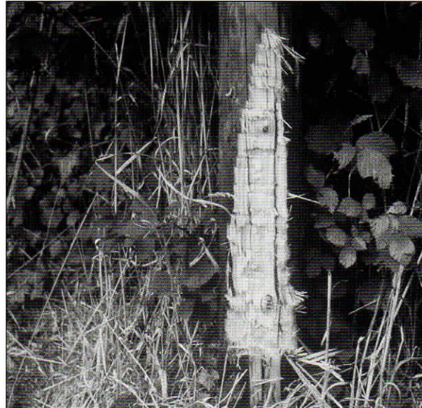
Figure 4. Mowing machine damage.
